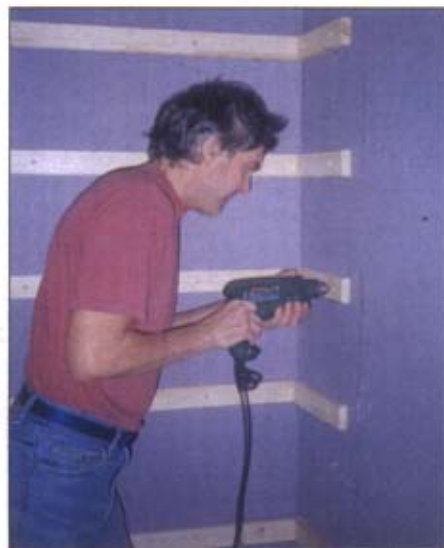
The shelf supports were first glued to the walls in the correct position, then drilled and plugged
