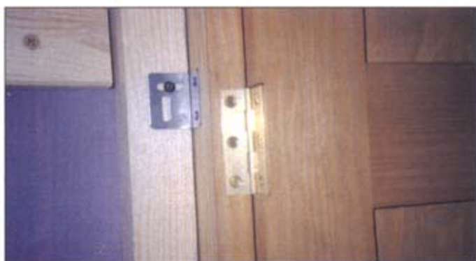
Using slotted plates to fix the frames to the wall battens allows some adjustment to be made to the frames to achieve the best fit for the doors
